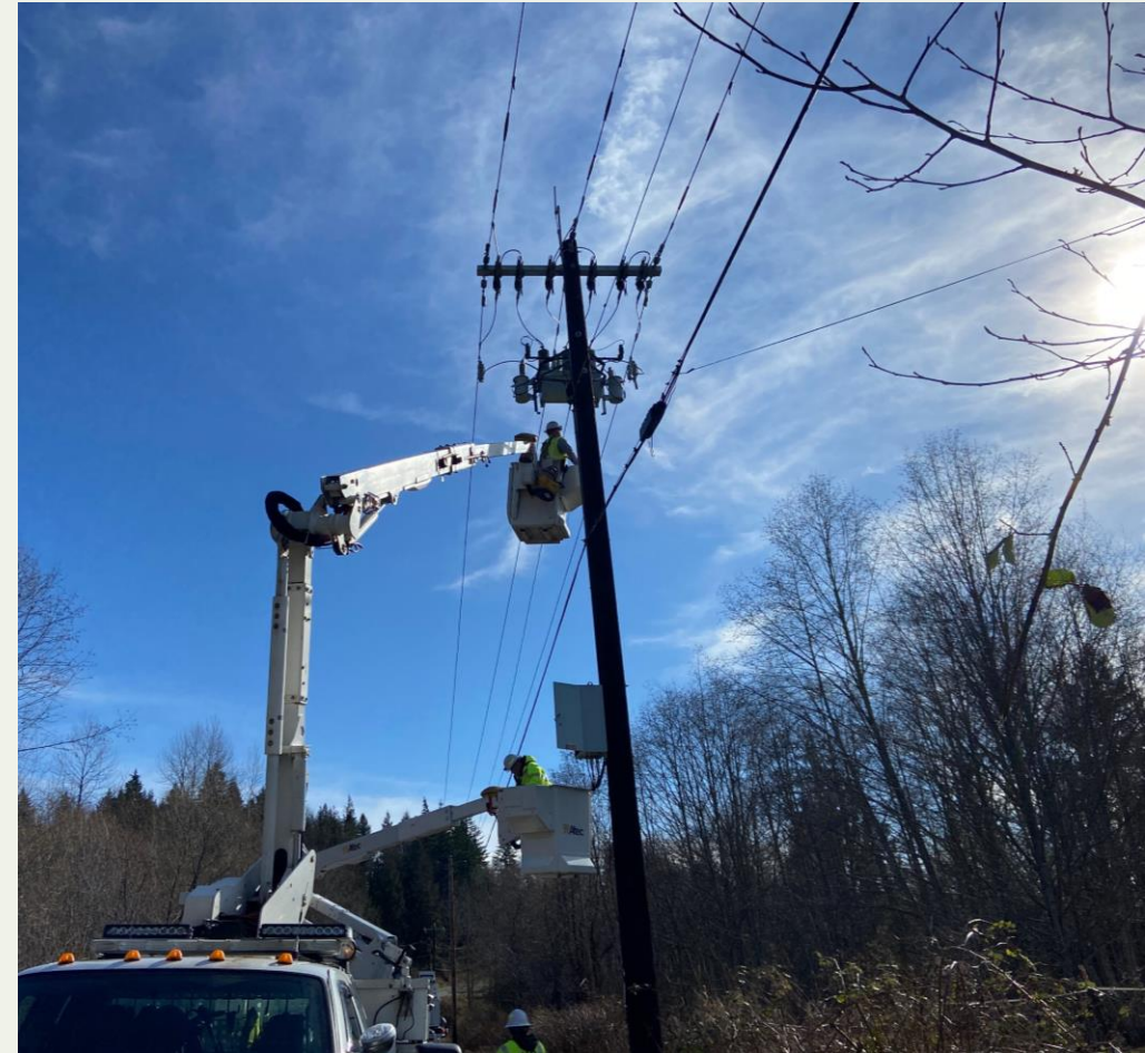
First DA Recloser commissioning in Arlington area as part of the project's proof-of-concept stage.
