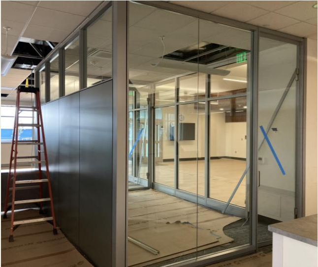
CSR Area- Conference Room Installation
