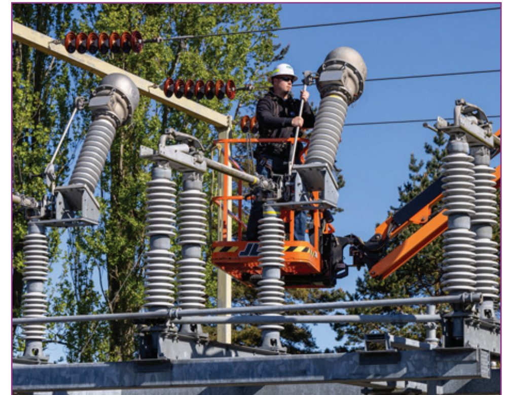
At the PUD, we're always working to ensure reliability for our customers. Here a worker breaks down components at the North Camano Substation May 2.
