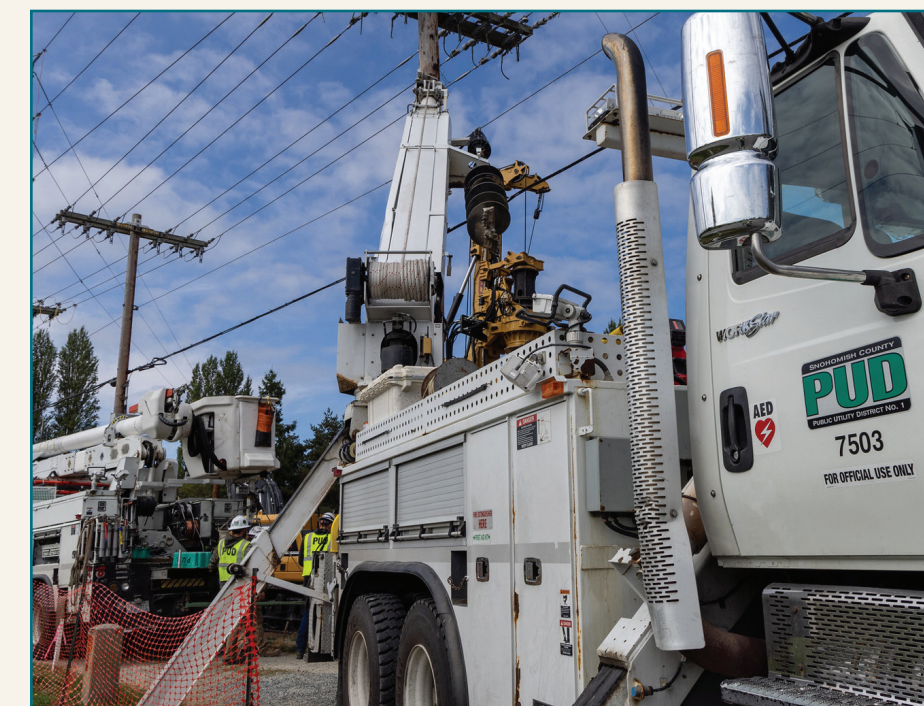
Summer also means construction and maintenance. As usual, the PUD was hard at it. Work included updates on a number of substations and pole replacements throughout our service territory.
